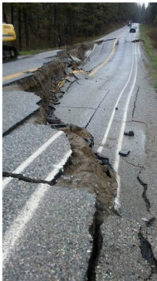
Inchelium Highway subsidence landslide, April 18 2017
