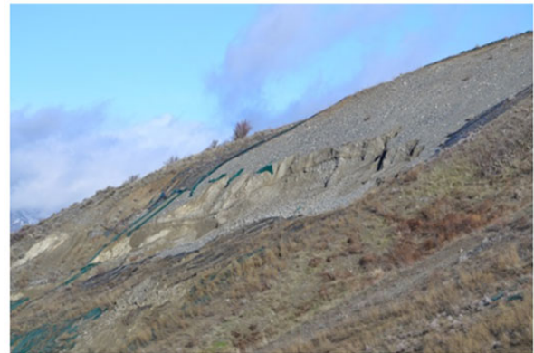
Upper slope failure, Mile Marker 1, Peter Dan Road, March 2017
